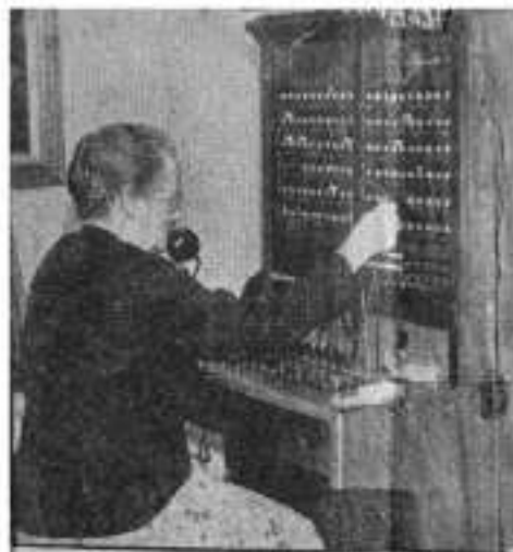
"Number, please." Mrs. C. Meddings, the village postmistress, plugs in for a call on the telephone switchboard, which is housed in her living-room.
